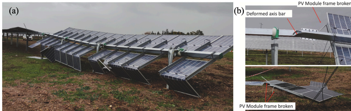
Fig. 11. Damage on a single-axis solar tracker due to wind-induced torsional load. Reproduced from Ref. Valentin et al. (2022) with permission from Elsevier, ©2022.
